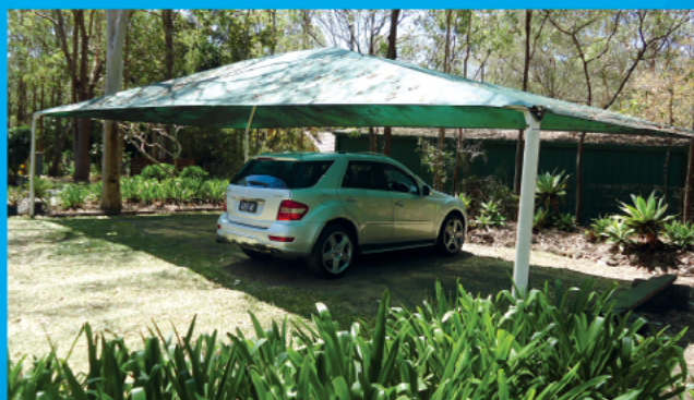
"15 Year old Z16 fabric conquers the harsh Queensland climate, installed in the Brisbane
